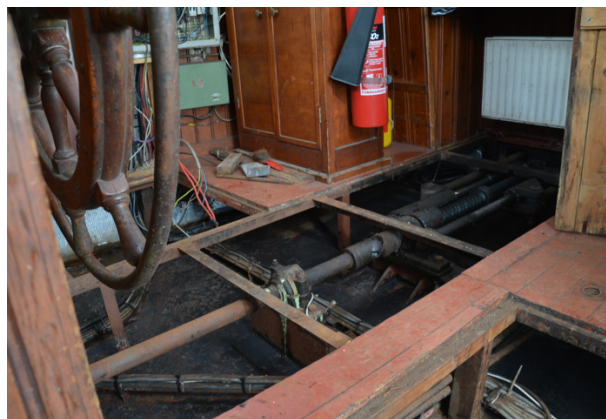
Wheelhouse floor removed for void cleaning and painting – showing rudder drive shaft.
