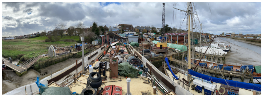
The Albatros is looking on first sight a little 'sad' with all her masts and rigging removed, decks littered with fixtures and fittings and areas been worked on.
