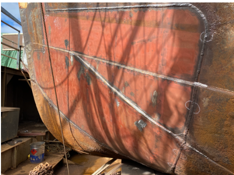
Insert plating to the front Portside Bow with welds following original plate lines
